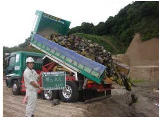
Fig. 10 Volcanic ash placed in a designated location (Photo courtesy of Kagoshima City Office)
